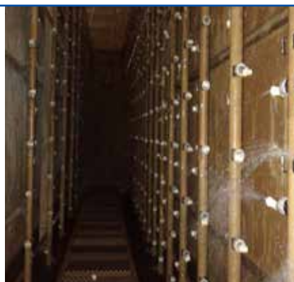
100% spray functionality due to clogged nozzles
