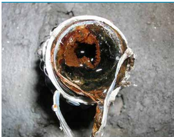
The pipe is almost clogged with scale.
